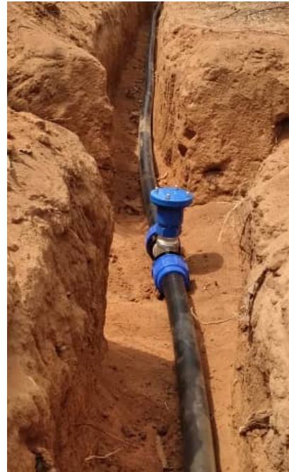
Above Distribution line in Mkutani
